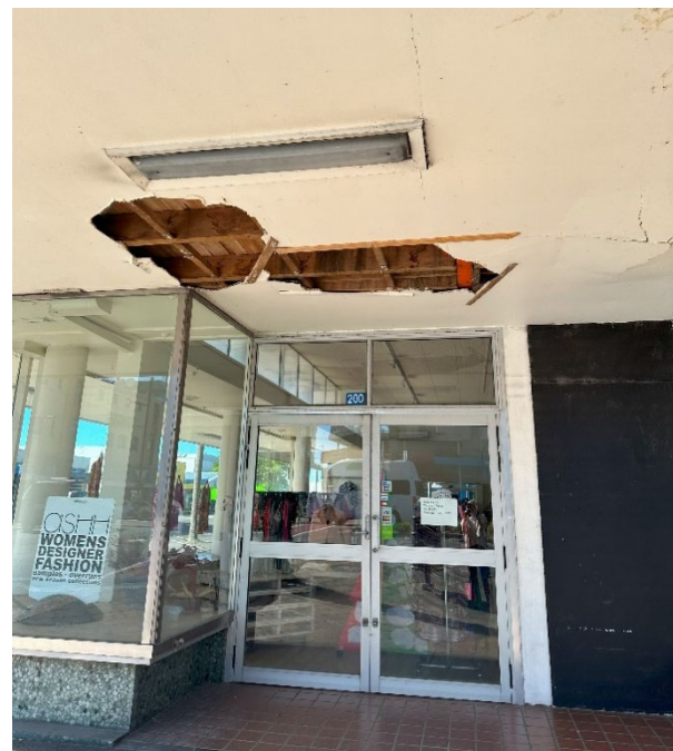
Main Street building decay. Gladstone Rd
