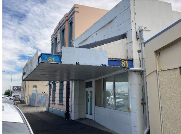
Deteriorating building. Childers Rd
