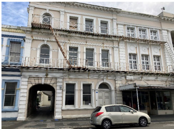
Masonic Hotel decaying façade. Lowe St
